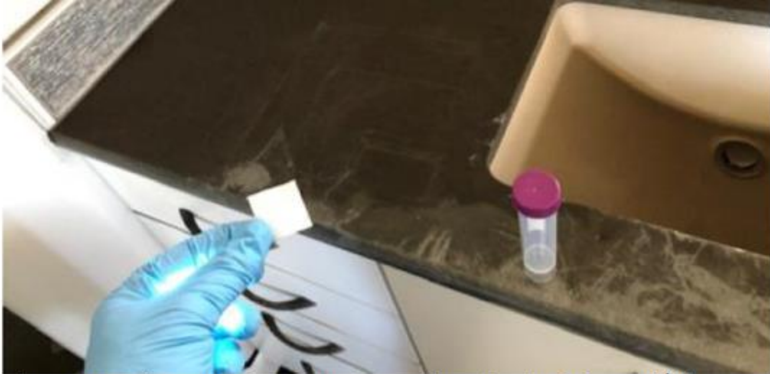
Photo 64: Wipe sample of smoke residue obtained from 2 nd floor master bath counters – held in file for possible future analysis
