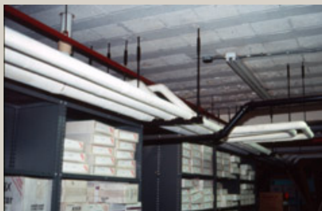
Overhead pipes with asbestos insulation
